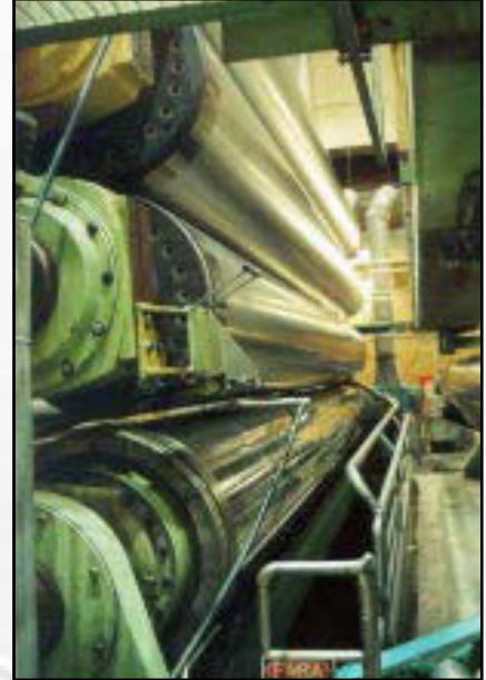
Calender stacks can be measured and aligned with the floor datum line as reference.
